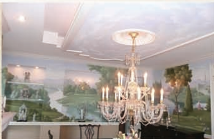
First Place -Glen Olsen, Jr. C.P., V&G Services, Woodbridge, IL and John Damme, C.P., Exquisite Interiors, Hickory Hills, IL 170 man hours installing Stark Tour du Monde panels to fit room layout
